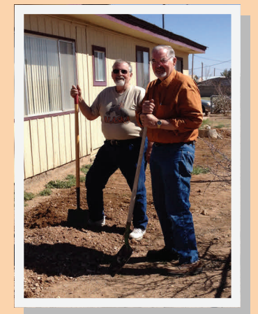
Bruce & Kris Lethin digging the electrical ditch for the Weaving and Fiber Arts Studio.
